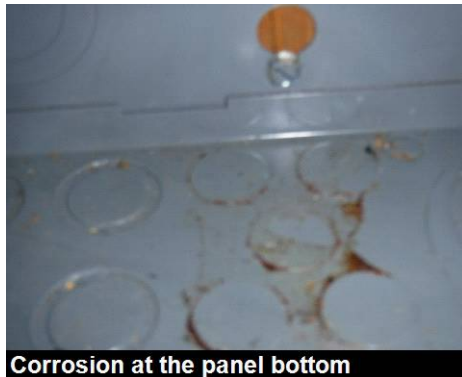
Corrosion at the panel bottom
