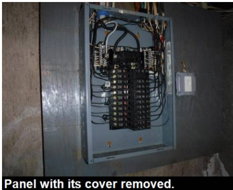
Panel with its cover removed.
