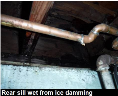
Rear sill wet from ice damming
