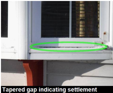
Tapered gap indicating settlement
