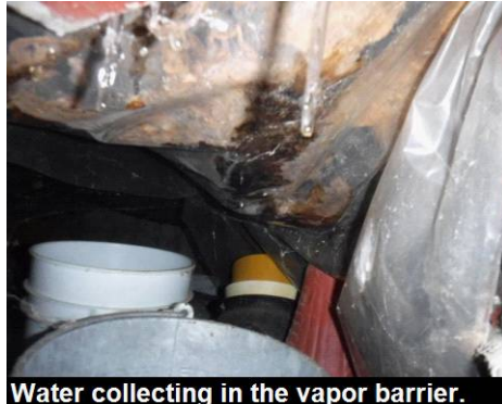
Water collecting in the vapor barrier.
